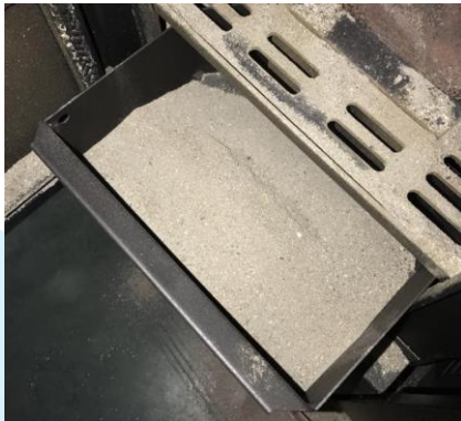
Example of dirty ash box
